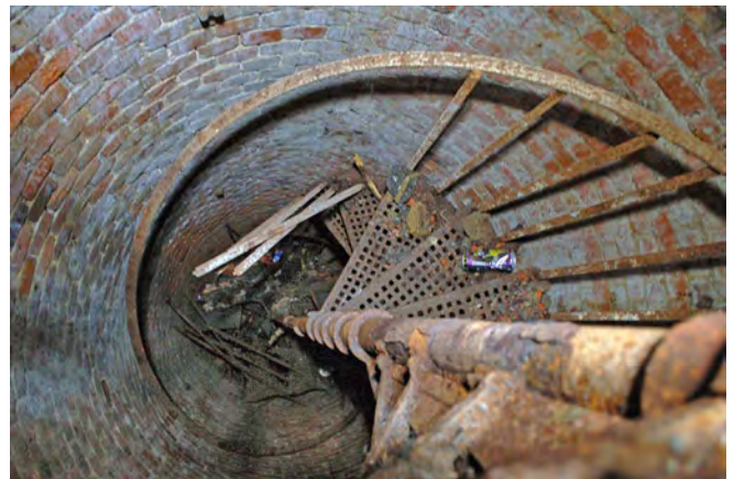
Recently ruined by repeated incursions, the bunker’s emergency stairs
